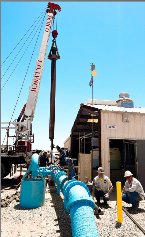
Operations Techs Brian Toner and Darren Dykes work on the repair at Well 8.
