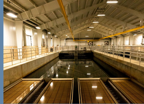
Water flows through the sedimentation basin at the treatment plant.
