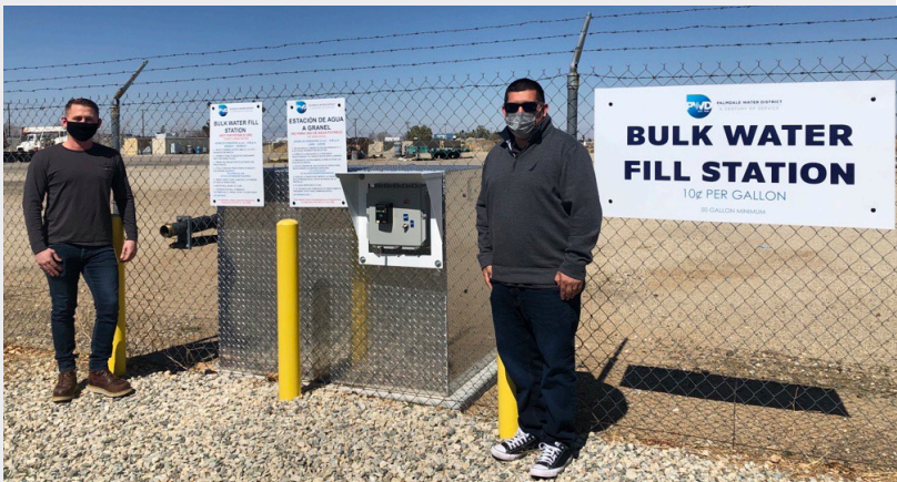
Assistant Engineer Jaron Hollida (left) and Engineering Tech Daniel Maldonado (right) checking the Bulk Water Fill Station.
